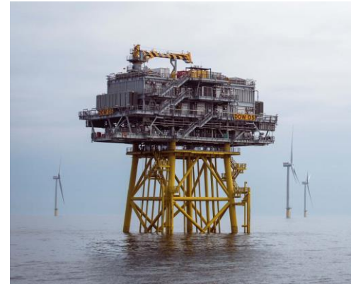
Dungeness offshore wind farm
