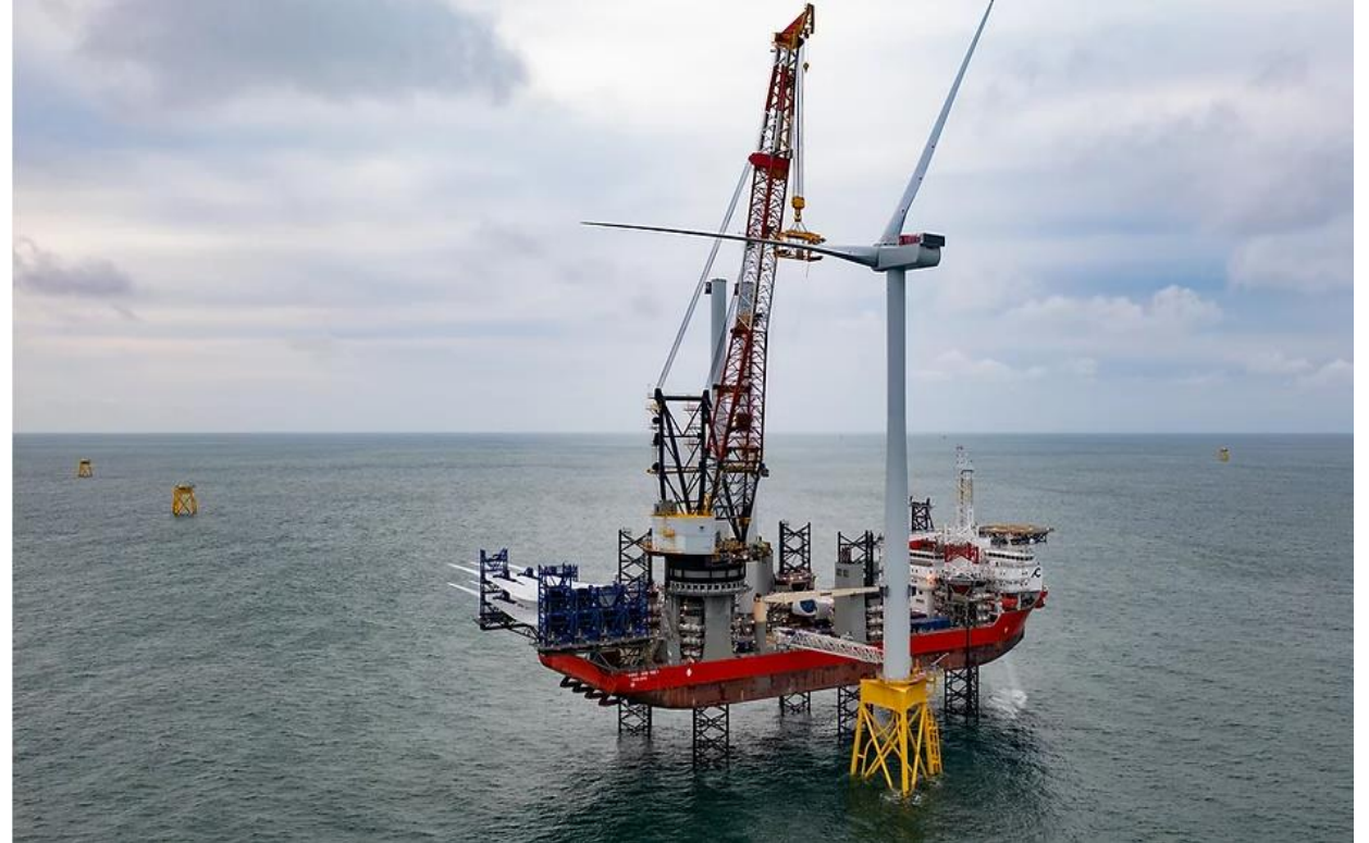
The Seagreen wind farm, offshore Scotland, uses jacket foundations in 40-60 m depth range (image: Seagreen Wind Energy)
